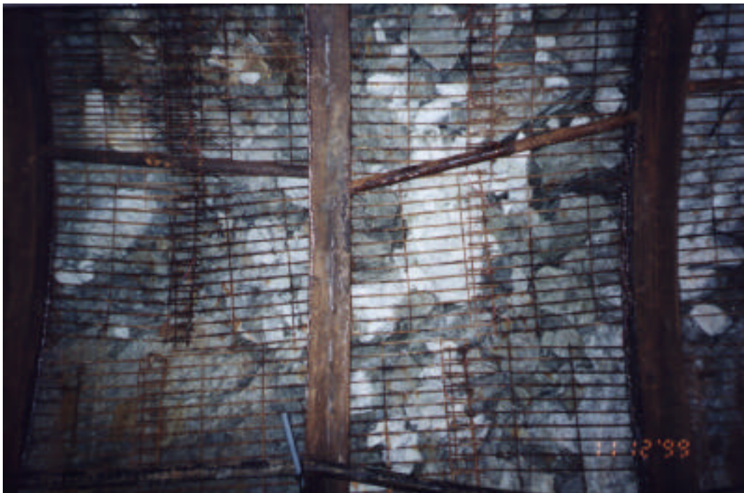
Figure 3. Photograph of Bloody Bluff Fault interval showing how the intersection of younger east-dipping fractures with older fractures has produced cobble-sized rubble requiring support of ring steel and wire mesh.
